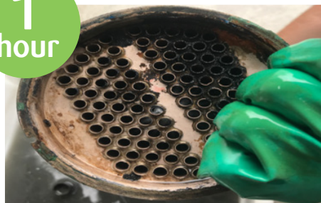
Volvo Heat Exchanger after 1 hour treatment of CleanScale.
